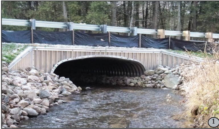
1. This open-bottom arch culvert allows species like the Wood Turtle to follow stream corridors safely while reducing the risk of road mortality. For an additional illustration of this structure, see Figure 10 in development techniques.
